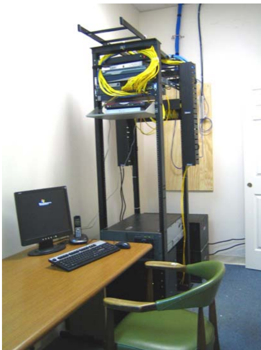
Electronics room (left) containing servers and communications equipment, and the hub for UMP's T1 communications link.
